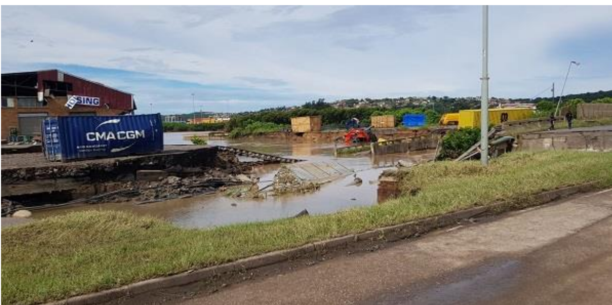
Flood damage to Bayhead Road, which gives access into Durban Container Terminal
